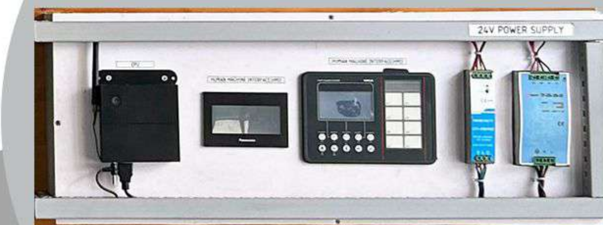
HMI / Power Supply
