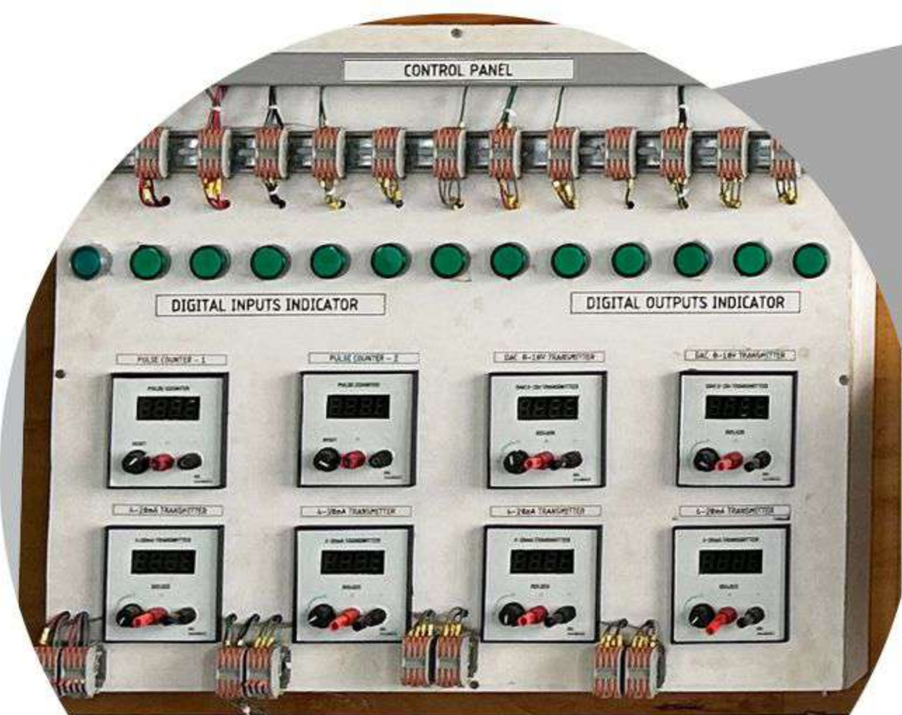
IO Control Panel
