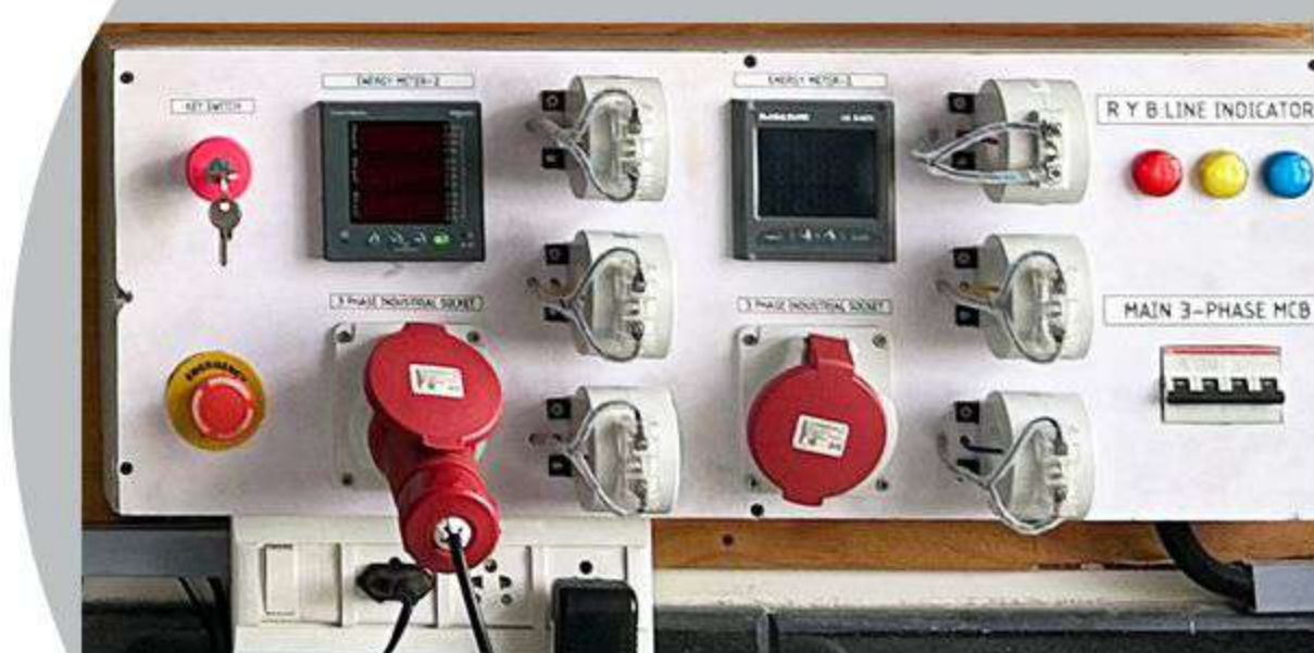
3 Phase Energy Meter with CT Coil
