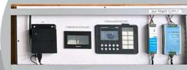
HMI / Power Supply
