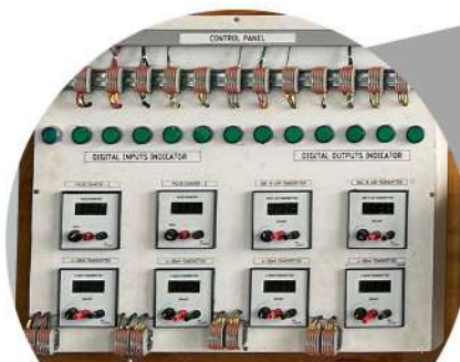
IO Control Panel
