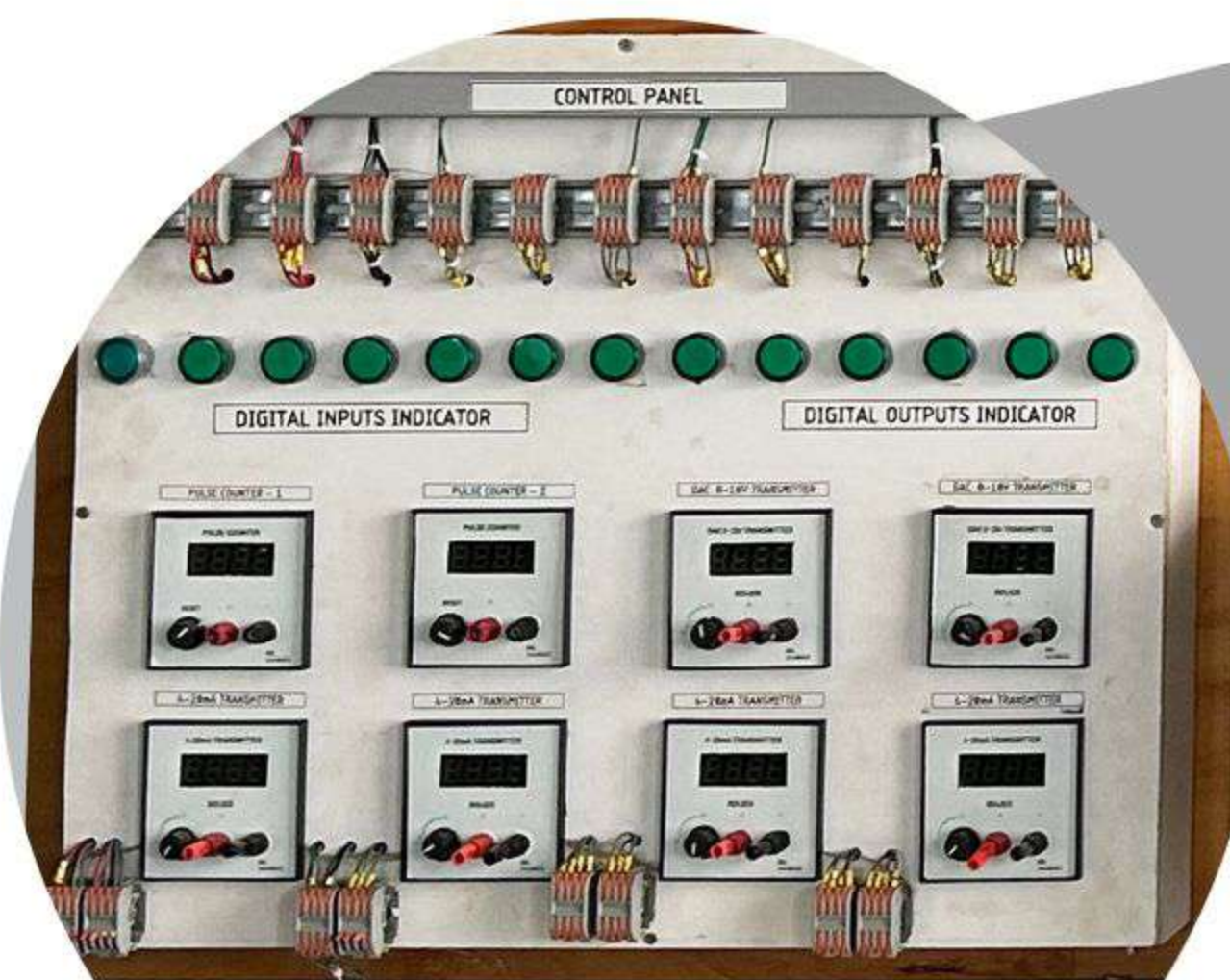
IO Control Panel
